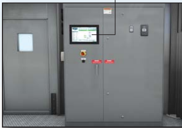
Main Control Panel – Interior View
